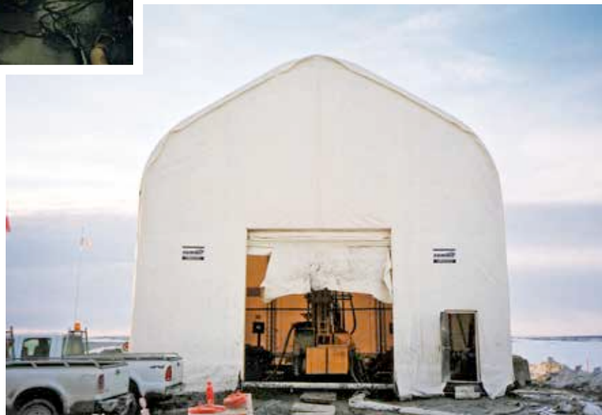
Fig. 6. Mobile shed for protection of the equipment and view of the machines at work inside the shed.
