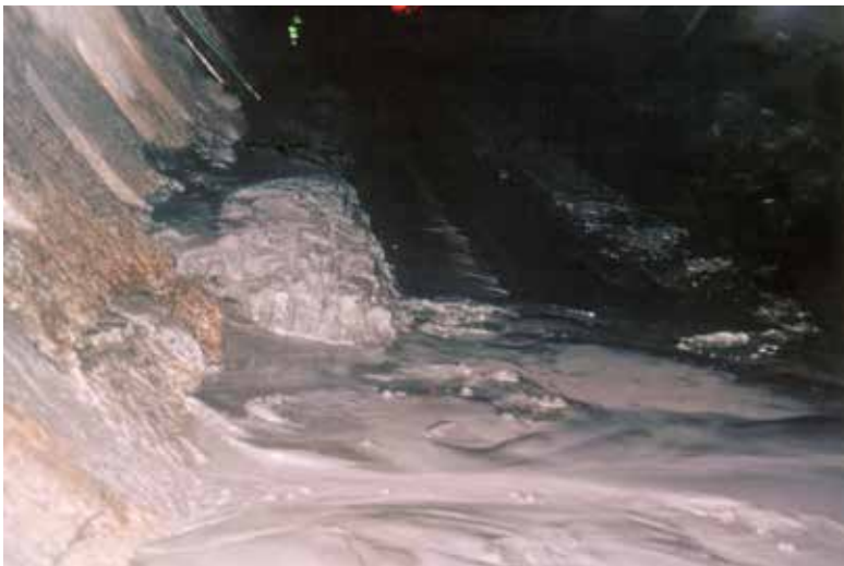
Fig. 4. Accumulations of material along the tunnel.
