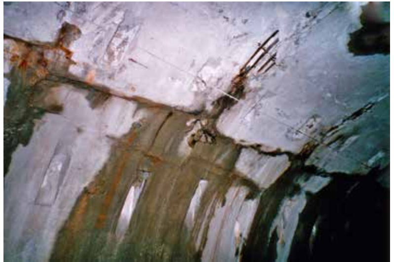
Fig. 3. Fissuring of slabs and water infiltrations.
