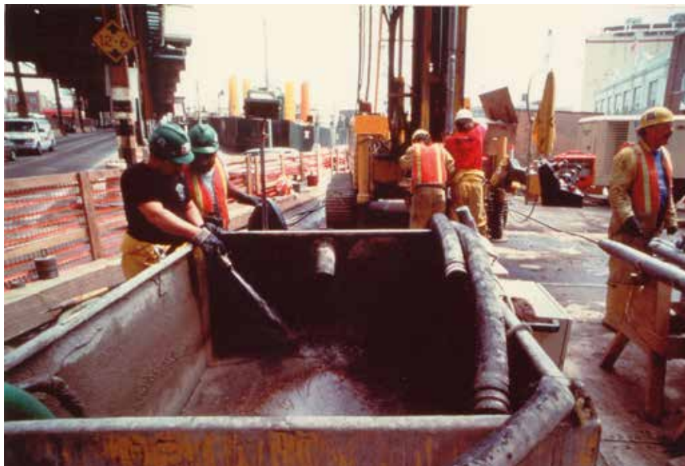
Fig. 6. Waste fluid collection tank.
