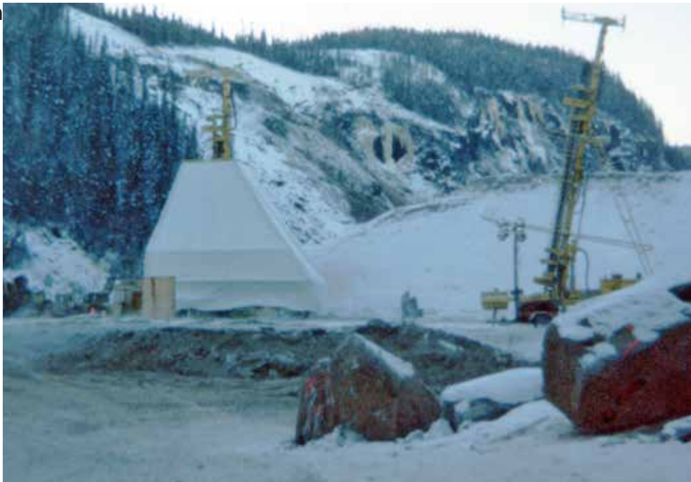
Fig. 7. P 1500 drill rig with removable cover for cold protection.
